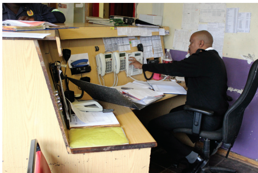
Victory Khanye fire services control room
